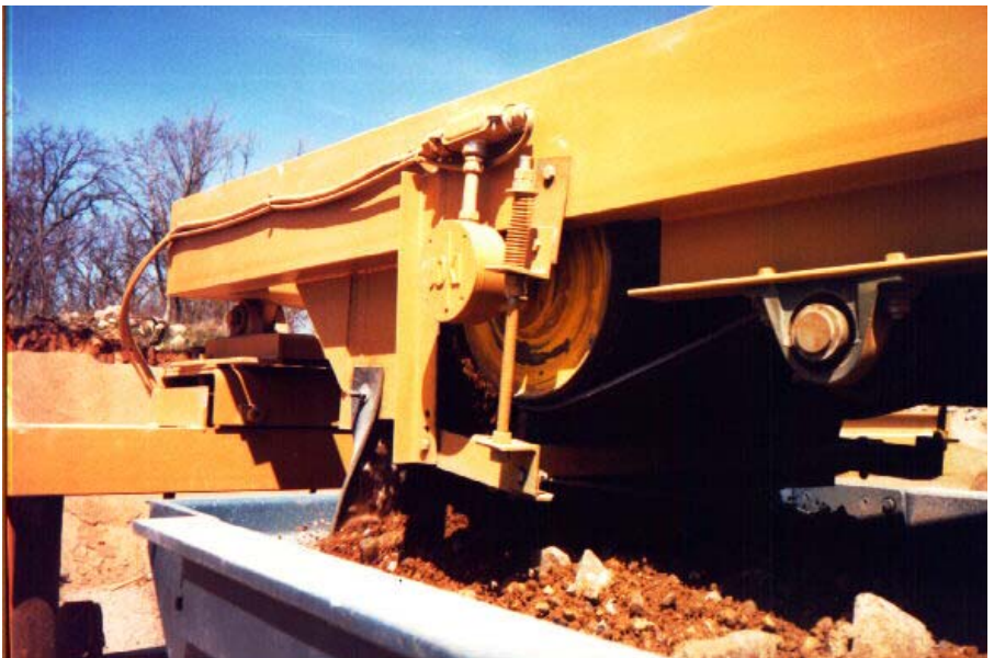
Fig. 9: Close-up of 15 HP elevating screen feed head drive pulley (in operating position.) Note optimal use of limited space. Motorized pulley was fixed to bottom of pivoting conveyor structure.
