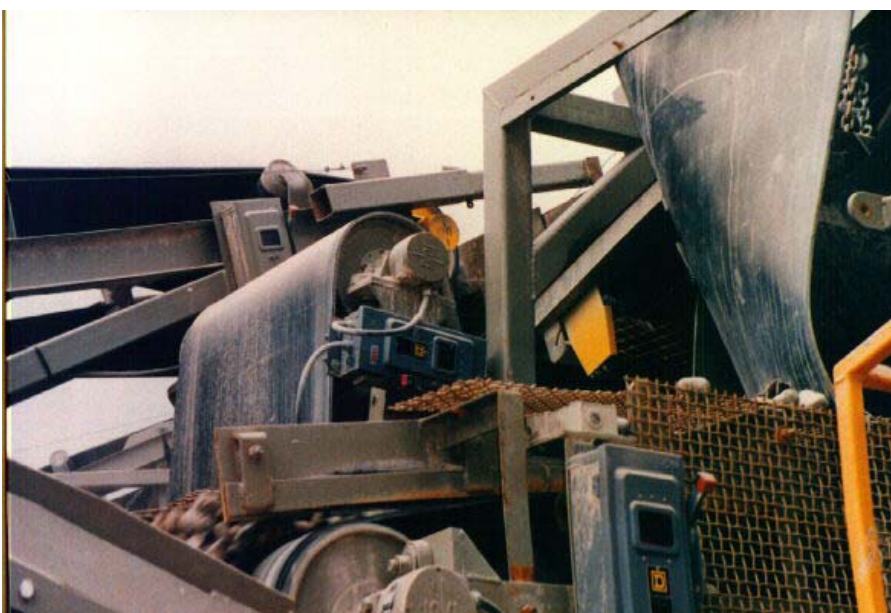
Fig. 5: Two 7.5 HP motorized pulleys in a congested area of a mobile crushing and screening plant installed in Ottawa, Canada in 1993. All motorized pulleys transfer heat into the conveyor belts they drive. Twenty motorized pulleys helped keep this facility operational throughout the bitterly cold Canadian winter of 1994.
