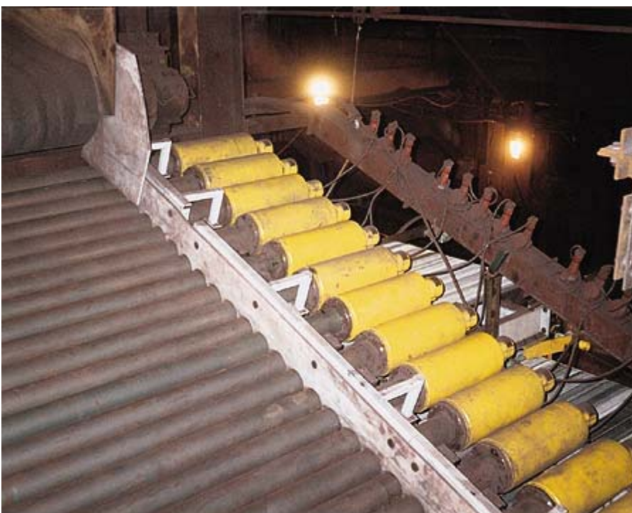
Fig. 14: Overview of 43 roller taconite pellet feeder after 1996 conversion to motorized pulleys. Engineering Design Services of Hibbing, Minnesota has now converted more than 150 feeder rolls for three taconite producers in the USA.
