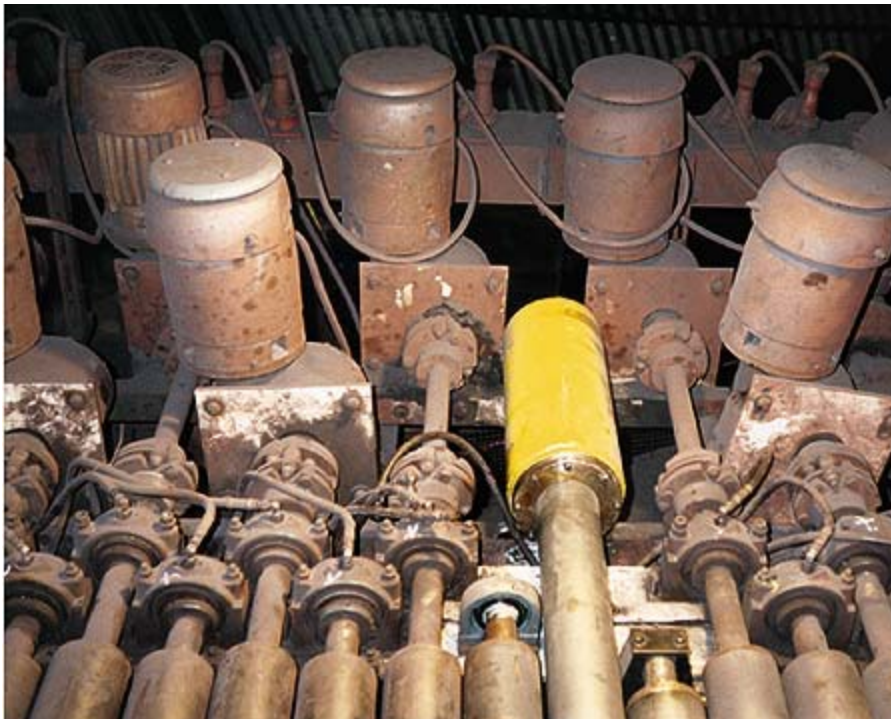
Fig. 13: Close-up of 1996 test of motorized pulley driving green taconite pellet feeder roll. Original German-designed equipment installed in Hibbing, Minnesota in 1972, included a motor, gearbox, jackshaft, two couplings, and three pillow blocks to drive each of 43 rollers.
