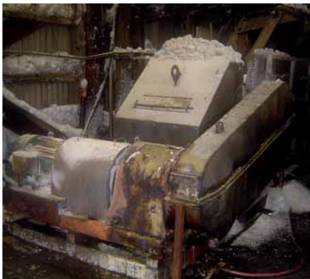
Exposed drive system for barge loading conveyor consists of motor, gearbox, chain & sprocket, all protected by cast iron and steel enclosures. Note steel enclosure built to protect personnel from rotating motor/gearbox coupling.
