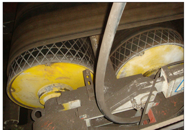
Two 75 HP Rulmecca Motorized Pulleys in "nested dual" arrangement move 1,200 tph of ROM coal at 600 fpm on 48" wide 1,200' long underground conveyor belt. Note the absence of external motor, gearbox, and pillow blocks. All mechanical components are hermetically-sealed within the pulley's oil-filled shell.
