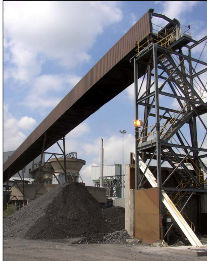
Figure 5 Kellingley Colliery replaced old problematic "bottom belt drive" near tail (left photo) on the main coarse discard conveyor in 2003 with 100 HP Rulmeca Motorized Pulley at discharge end above pile (right photo) and eliminated 300,000 tons of lost production annually.
