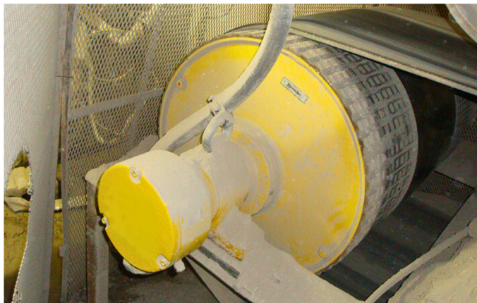
Figure 4. Motorized pulley installed in reclaim tunnel subject to flooding. Note partial lagging on outer thirds of pulley shell.
